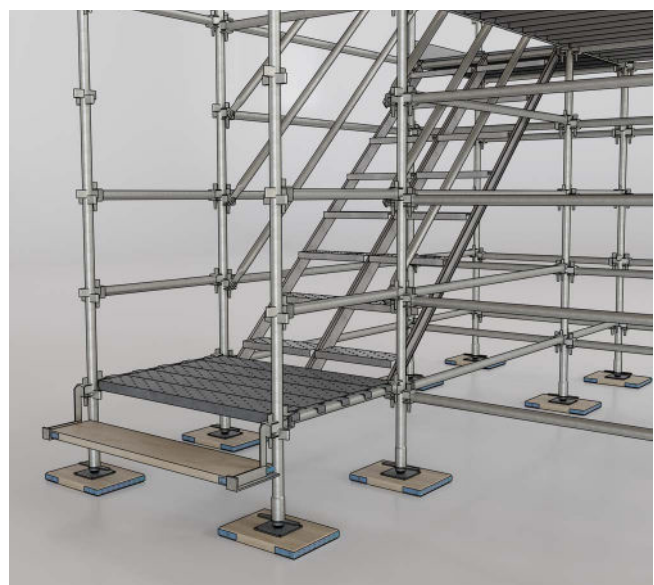
Figure 20: An example of stretcher stairs
