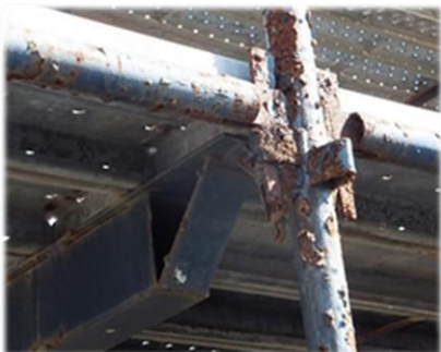
Figure 9 Severe corrosion on critical scaffolding components
